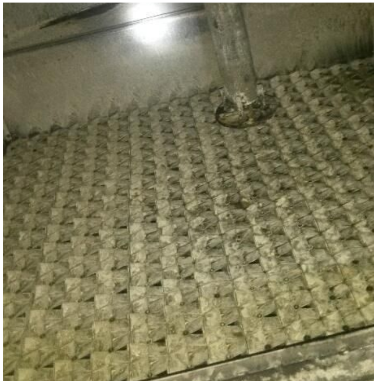
Figure 3. The multi vortex wet scrubber dispersive grating after one year of the continuous air treatment process. The gaps in the grating elements are clearly visible.
