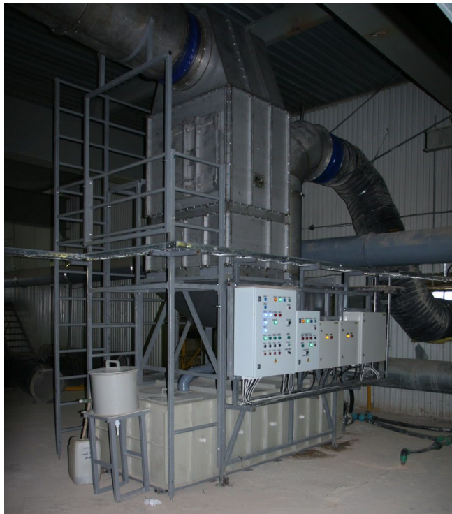
9,500 cfm multi vortex wet scrubber chamber installation at the Polymetal Corporation facility
